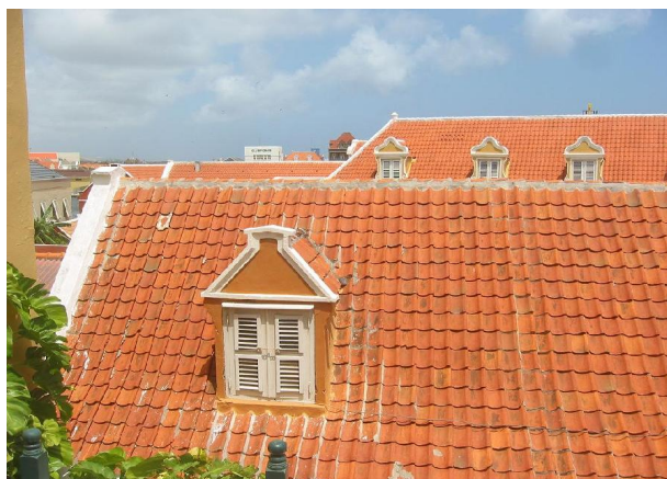
Orange clay-tiled roofs fill the horizon as viewed from the balcony of Kura Hulanda Museum
