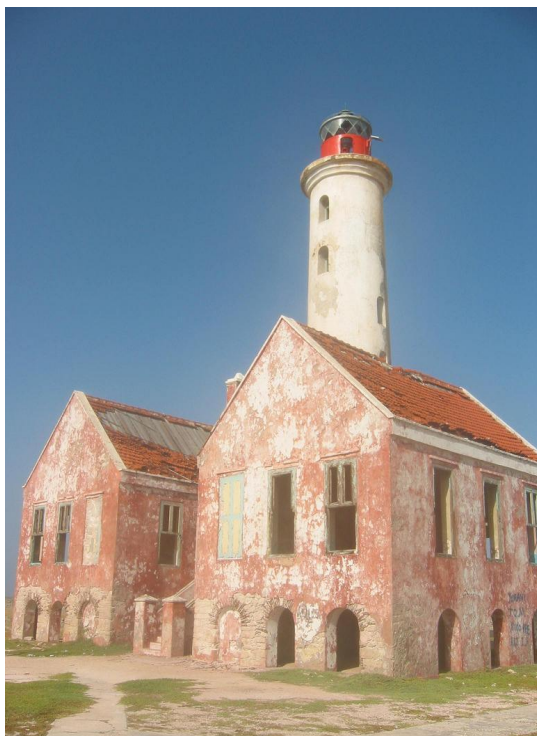
Klein Curaçao lite – Though dilapidated, the circular climb up the steps of the Curacao lighthouse was worth the climb.
